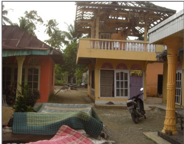
(Far left) Ifel with son Razia stares into a daunting future (Left) All three houses severely damaged
